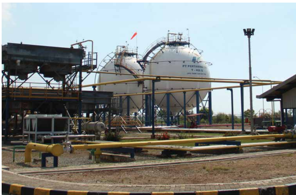
One of the LPG Tank facilities owned by Pertagas to support the availability of national LPG need.
