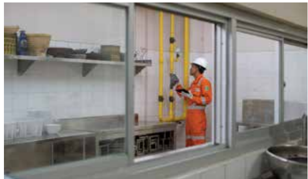
To ensure the safety and reliability of gas distribution, PGASSol staff routinely carry out operations and maintenance of natural gas infrastructure facilities.
