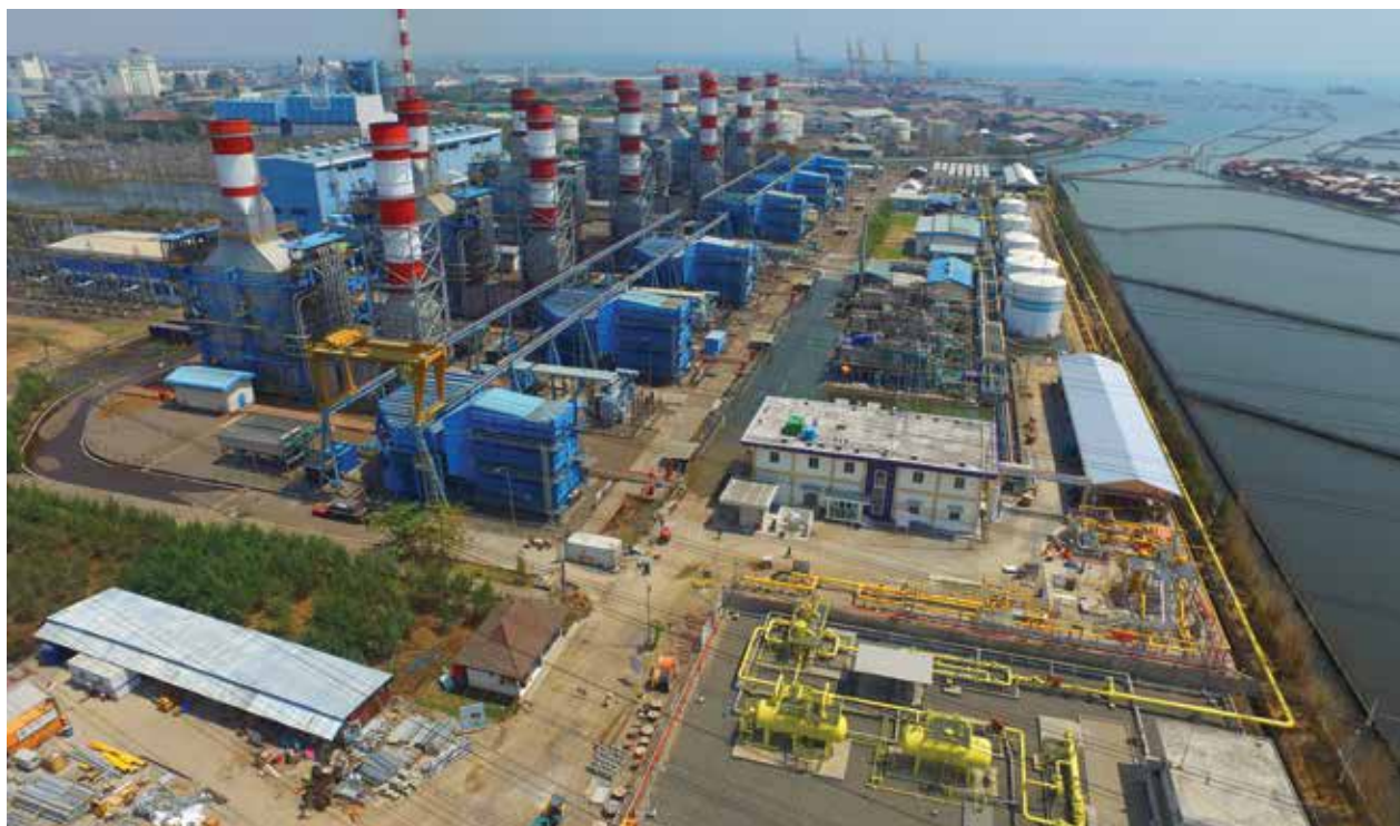
The KJG station facility is operated to supply gas to PLN Tambak Lorok in Semarang - Central Java.
