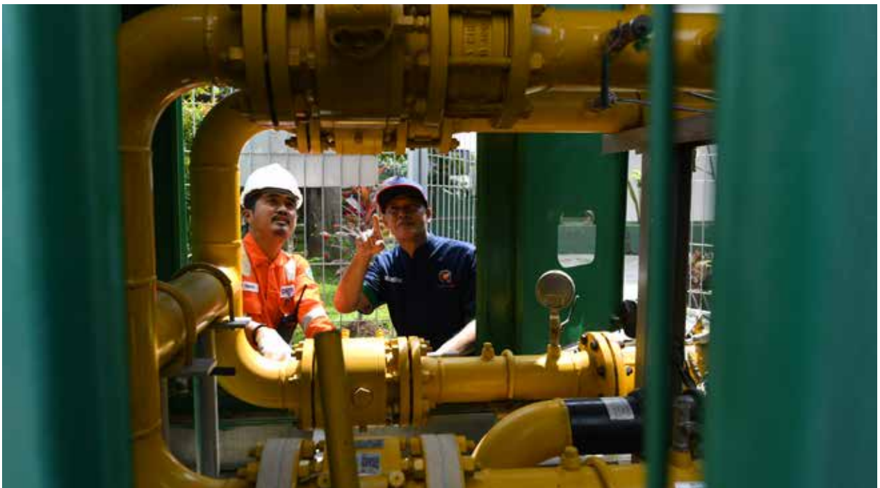
MRS Maintenance Activities are carried out to ensure the safety and reliability of gas distribution.
