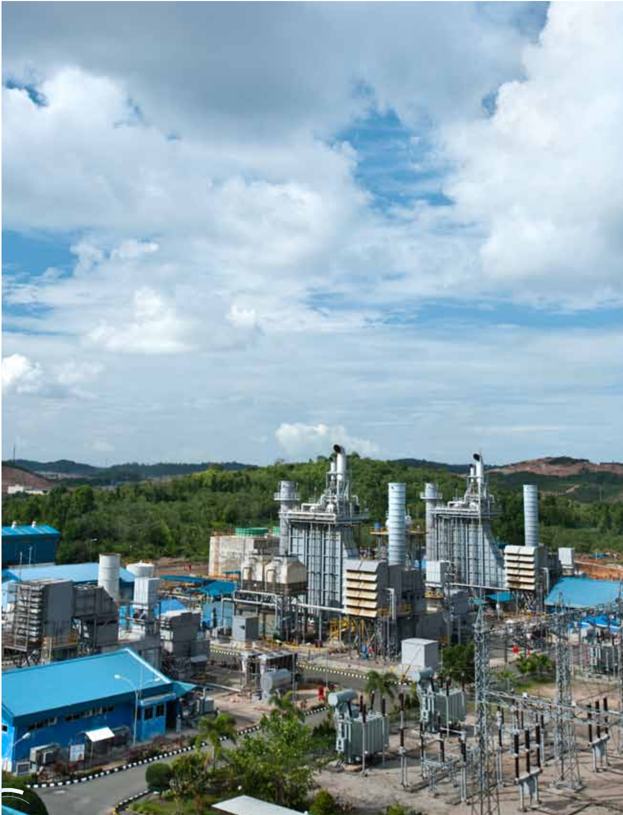
PT Dalle Energy is PGN's largest customer in Batam, using natural gas for its non-PLN power.
