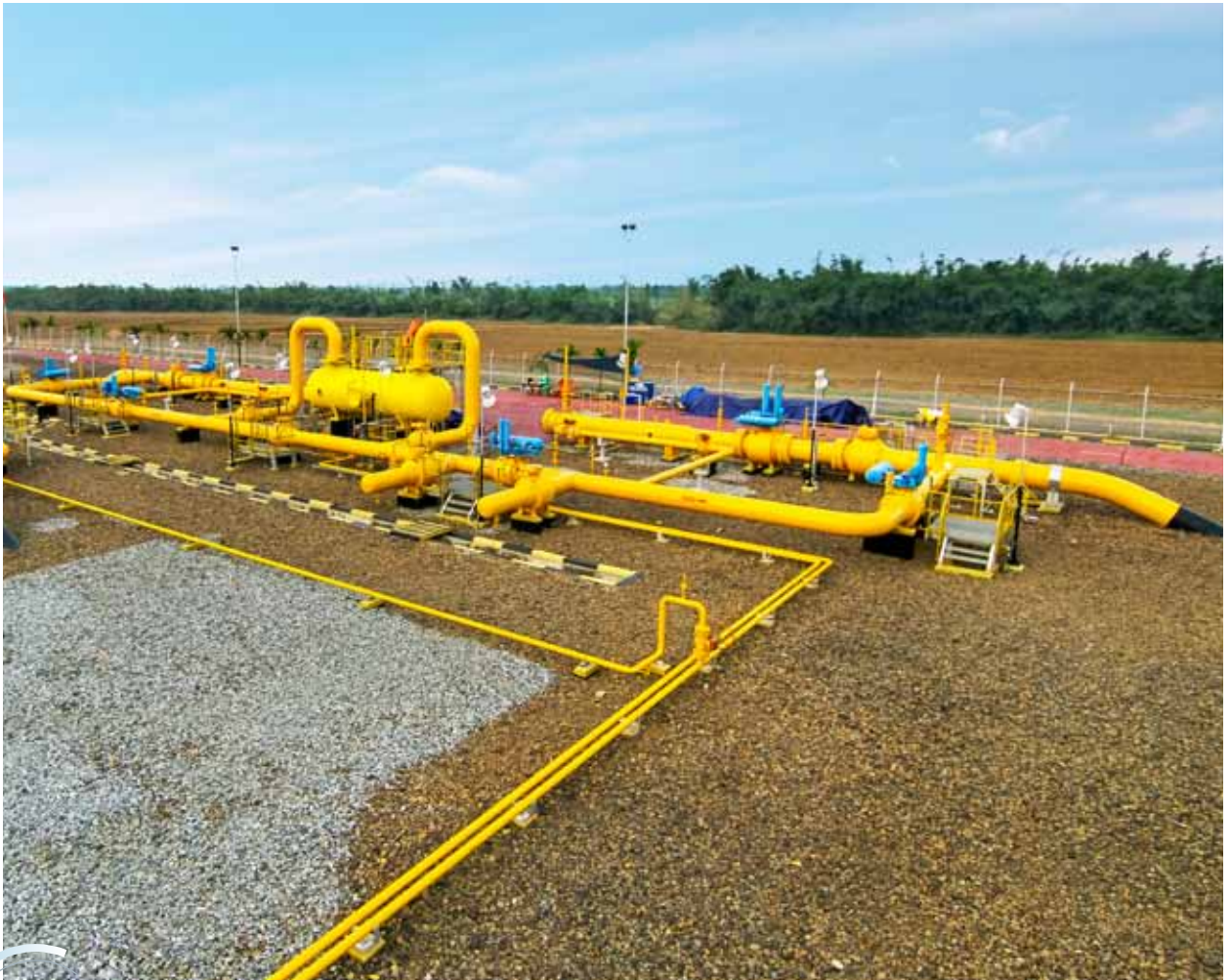
Gas Station Terbanggi Besar located in transmission pipeline SSWJ (South Sumatera West Java) Kilometer pipeline 171.3, constructed in Lampung Province, Sumatera. With area 16 Ha, this station functions as a pressure and temperature control to ensure smoothness and safety in transporting gas. It was developed in 2005 and became operational in 2007.
