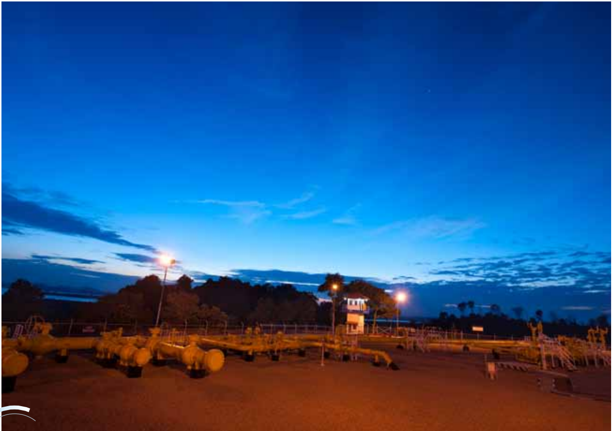
Gas receiving station belonging to PT Transportasi Gas Indonesia, a subsidiary of PGN, in Panaran, Batam
